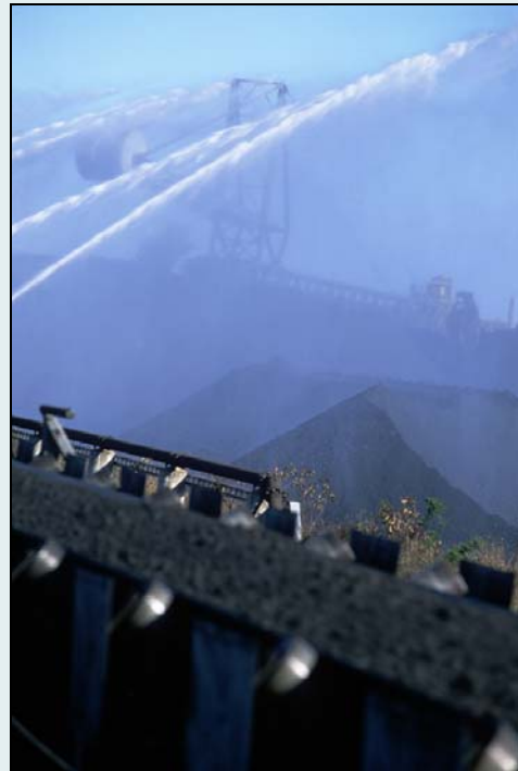
The stockyard's 156 water sprays are controlled by an automated system connected to real-time weather monitoring stations.
